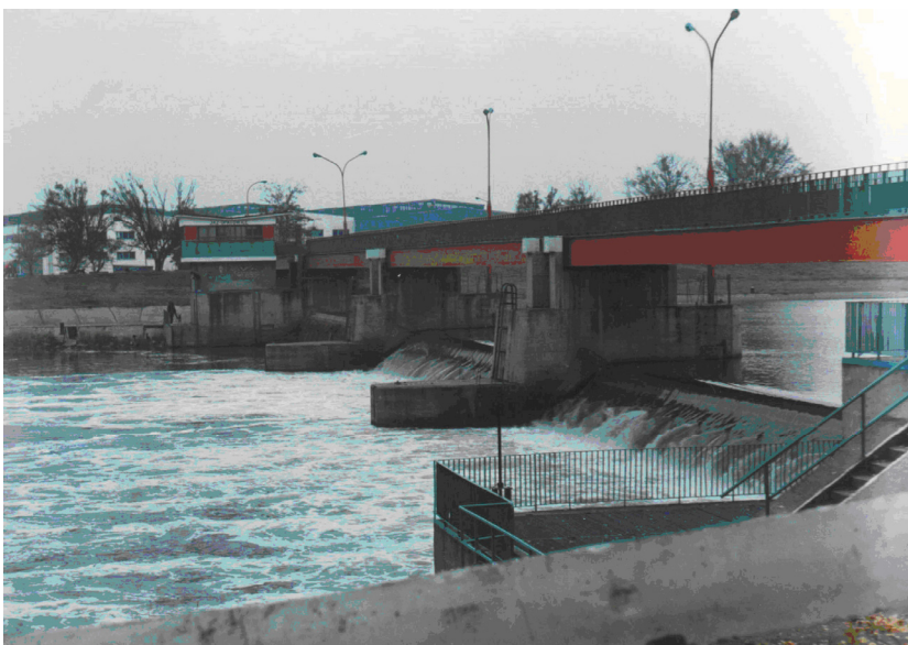
Figure 9. The moveable gate structure at Opatowice upstream of the town of Wroclaw
