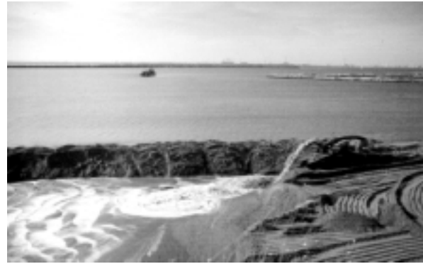
Fig. 3. Nourishment works on Aculadero beach, with the pipeline pumping sediment on to the beach. Note the dredging boat in the background.
