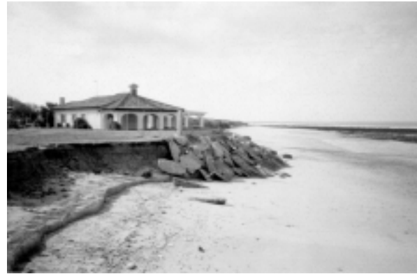
Fig. 2. Erosion problems near Punta Candor. The Quaternary cliff is eroded and summer houses are protected by a rip-rap revetment.
