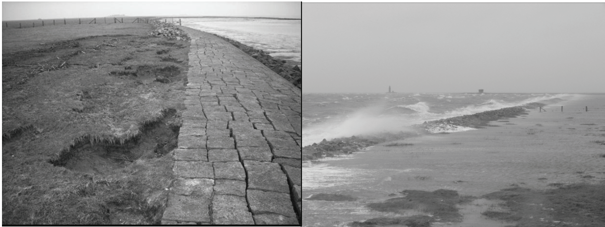
Figure 1: Scouring at the existing revetment (left), overtopping during storm tide (right) (Photos: N. Kumbruck).
