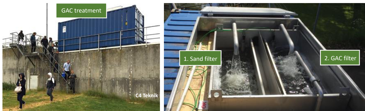
Figure 23. Pictures of the GAC filter at Kristianstad WWTP taken during the MORPHEUS study visit in May 2017. The removal of selected indicator MPs is shown in Table 17. Photo: Erland Björklund.
