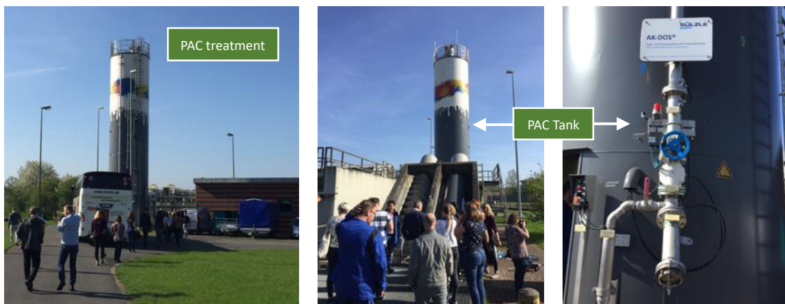
Figure 16. Pictures of the PAC system at WWTP Dülmen in Lippeverband, taken during the MORPHEUS study visit in April 2018. The removal of selected indicator MPs is shown in Table 12.
