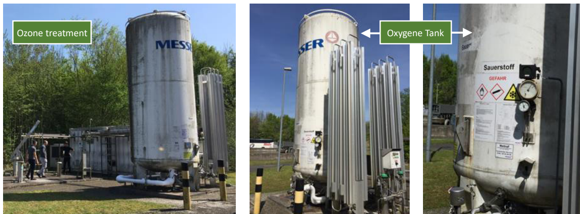
Figure 14. Pictures of the ozonation system at WWTP Bad Sassendorf in Lippeverband, taken during the MORPHEUS study visit in April 2018. The removal of selected MPs' indicators is shown in Table 11. Photo: Erland Björklund.
