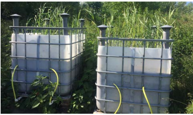
Constructed pilot plant of RBS at WWTP in Swarzewo: two cubic pilot plants RBS (August 2020), photo: A. Kupczyk
